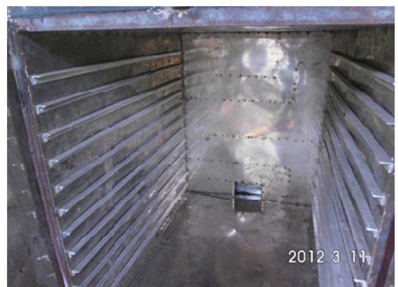
Figure 3. Inside the chamber of the rice hull-fueled dryer
